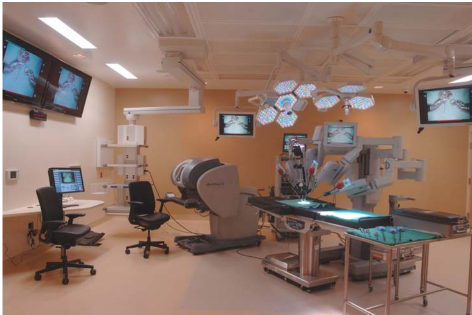
Black Diamond Video's IDSS system installed in a surgical robot-equipped operating room at Saint Francis Hospital and Medical Center.
